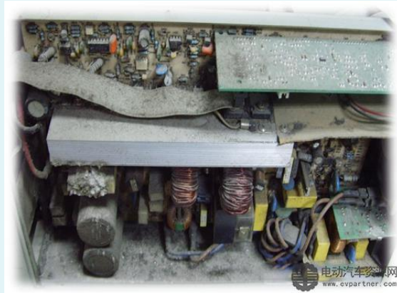
Non-separation duct power module 2-3years later inside
